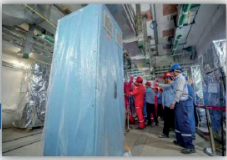
DCS Installed and Commissioned March 31, 2024
