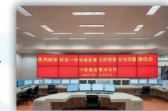
Main Control Room Operational May 21, 2024
